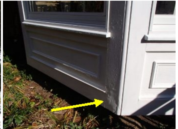
wood is patched, soft
