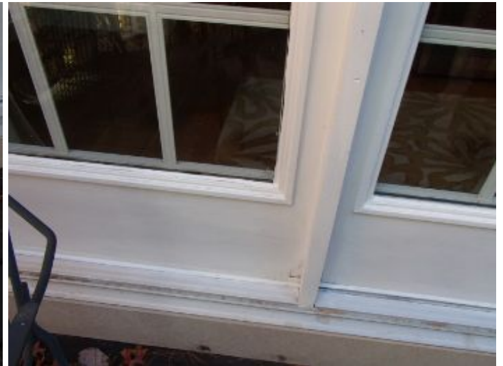
painted over water damage
