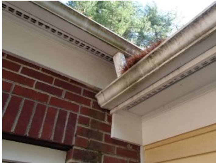
gutter backing up against siding
