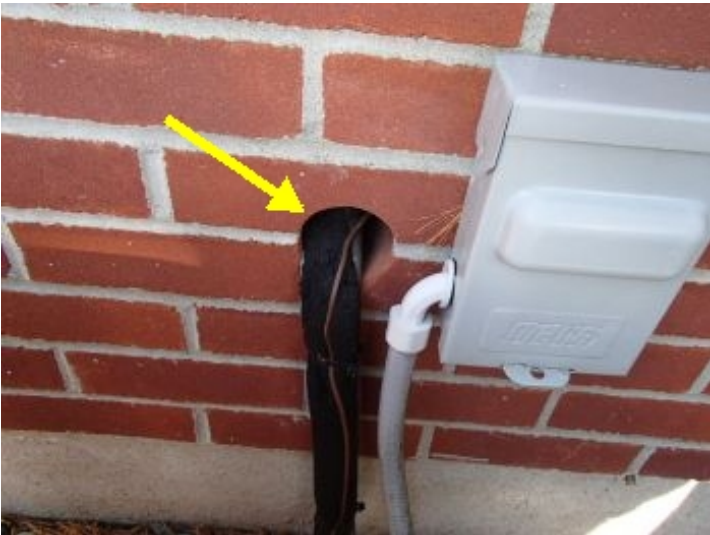
2 ac line holes allow vermin entrance
