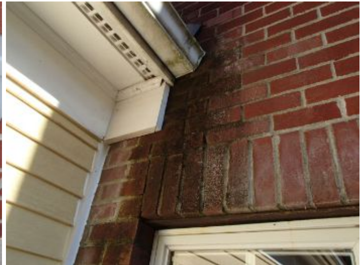
gutter water damaging brick
