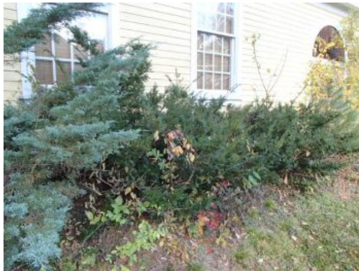
area where foundation is bowed, no gutters, vegetation
