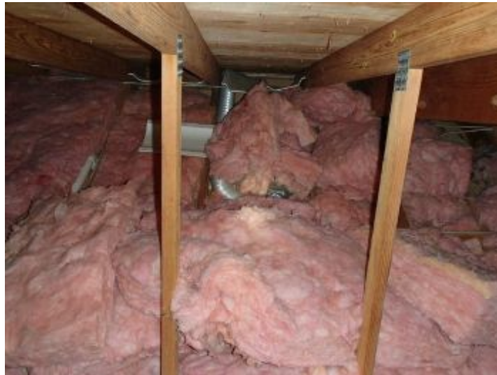
garage attic bathroom venting in soffit
