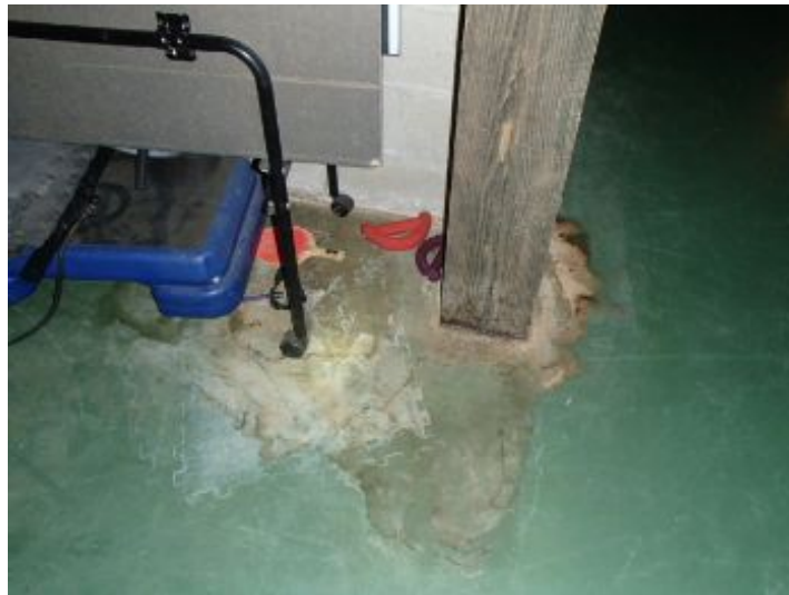
leaking chimney in basement from cleanout
