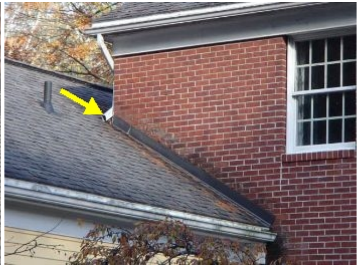
termination on the roof, overwhelmed gutters
