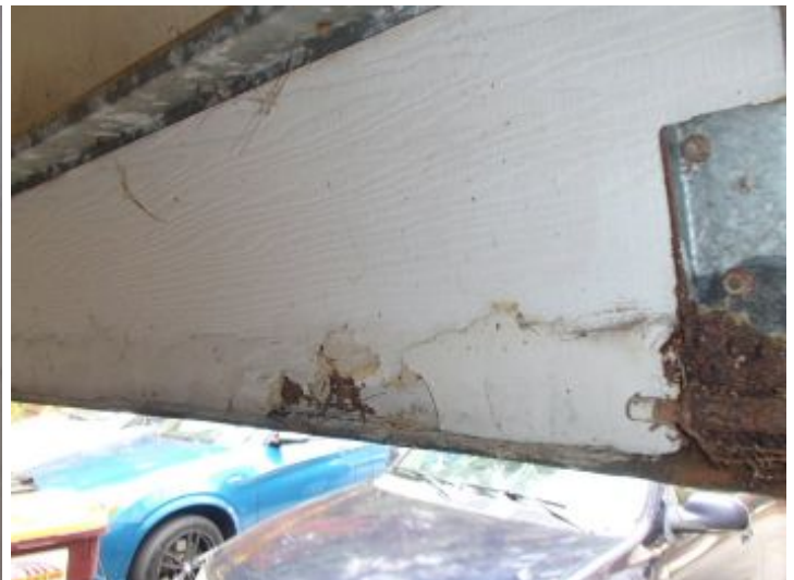
corrosion, rot on door
